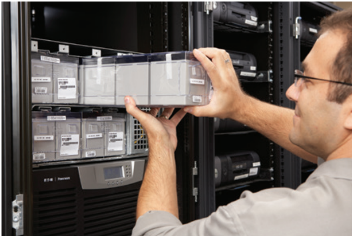
IT staff can easily replace battery modules.
