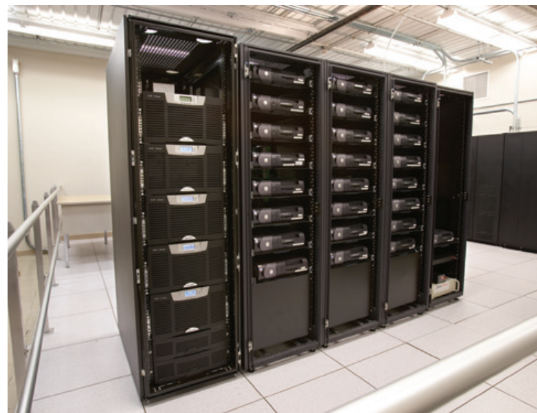
The BladeUPS remains cool even in a data center full of servers.
