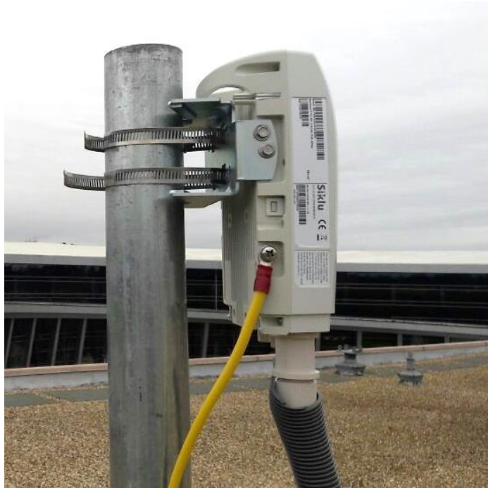
Figure 3: MultiHaul™ T200 installed
